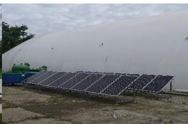
Figure 2. Photovoltaic system for energy production
