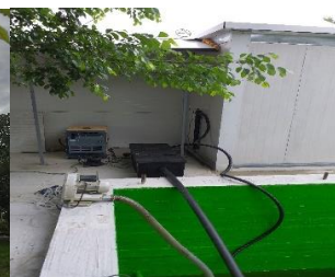
Figure 4. Aeration system and diesel generator
