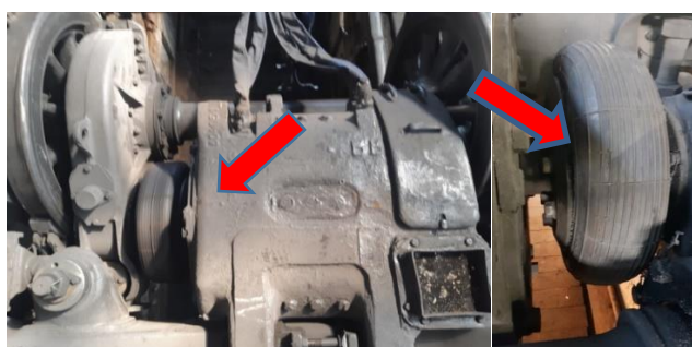
Figure 3. Place for equipment with shock-vibration sensors
