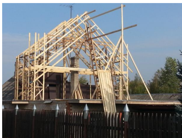
Figure 3. Construction of the experimental object roof structures level transition what give it an attractive appearance and creating double strength in to roof middle area
