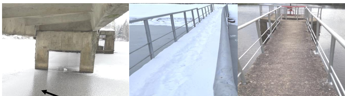
2 pav. Priežiūros tiltelio pasvirusi perdanga Fig. 2. Deformations of service bridge plate
